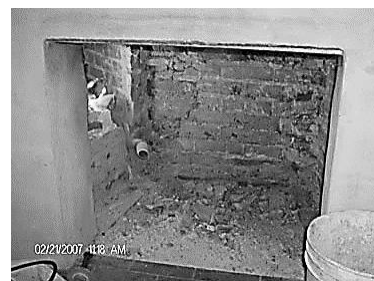
Badly Deteriorated Firebox
