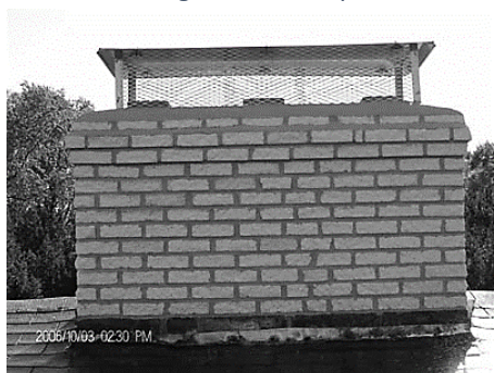
Metal Cap on Clay Liner Chimney Top
